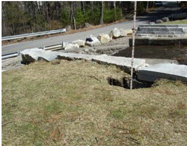
This two-foot sinkhole was created by last March's rains.
