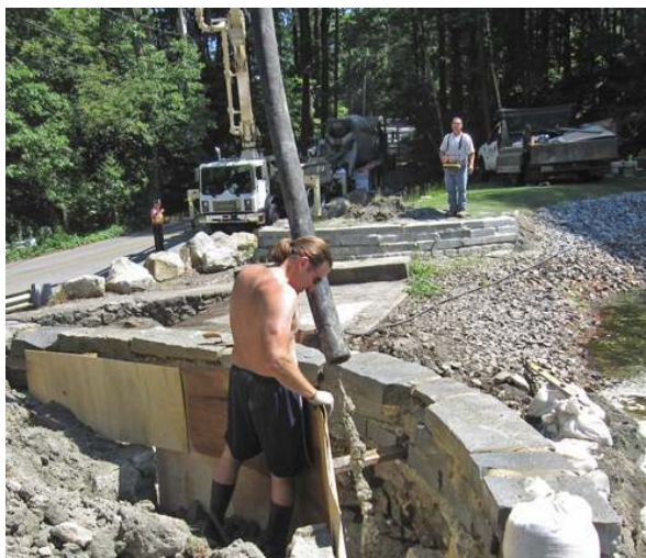
Seven cubic yards of concrete, pumped from equipment on Rattlesnake Hill Road, fortified the dam's most vulnerable flanks.
