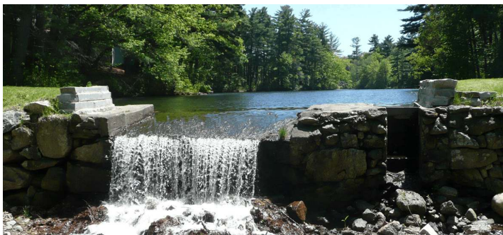
Hundreds of hours of volunteer labor enhanced the safety of the Foster's Pond Dam. The granite on both sides of the picturesque spillway allow the dam to handle high water without overtopping the earthen crest.
