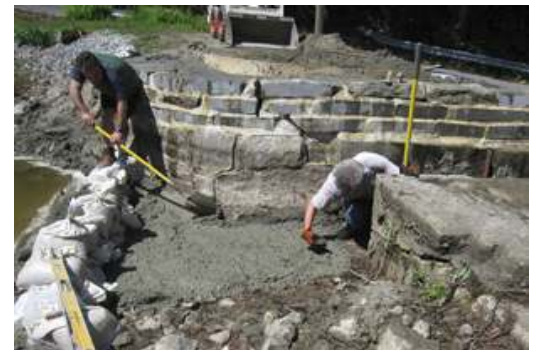
The Pond was kept low last summer so that leaks in the sluiceway could be repaired by neighborhood residents.
