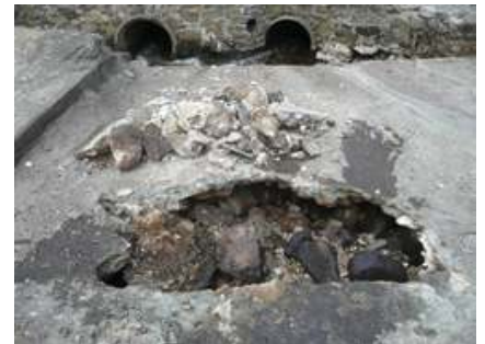
It took two tons of concrete to fill this cavern under the spillway after the March flooding.
