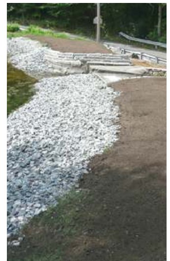
Tons of loam and crushed stone went into finishing the work last Summer.
